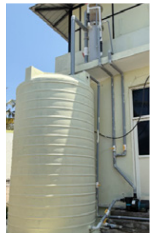
Seawater filtration facilities
