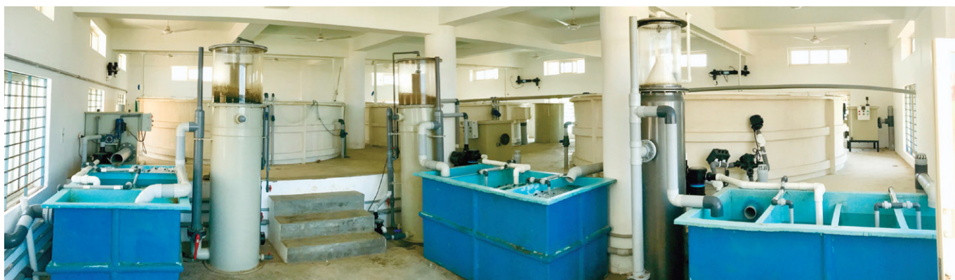
RAS facility at Vizhinjam Research Centre
