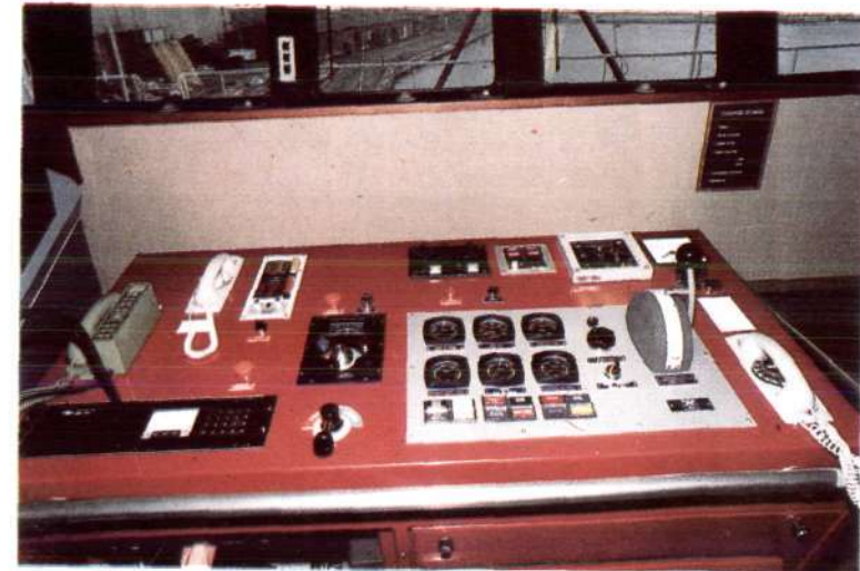
Wheel-house control panel
