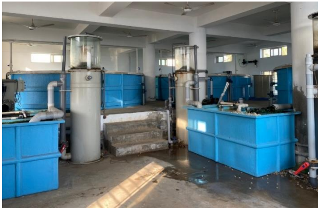
RAS 30 t Brood fish rearing tanks
