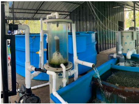
10-ton RAS fingerling rearing unit at Thrikunnappuzha
