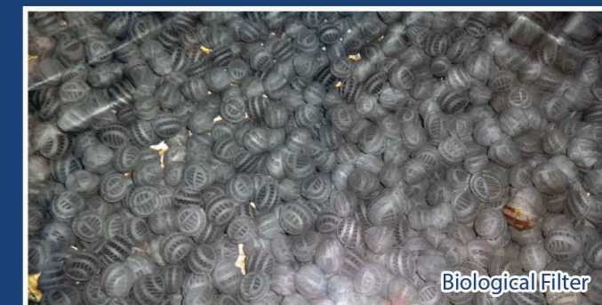
View of biological filter in RAS
