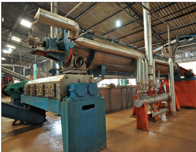
Plate 12. Interior view of fishmeal plant
